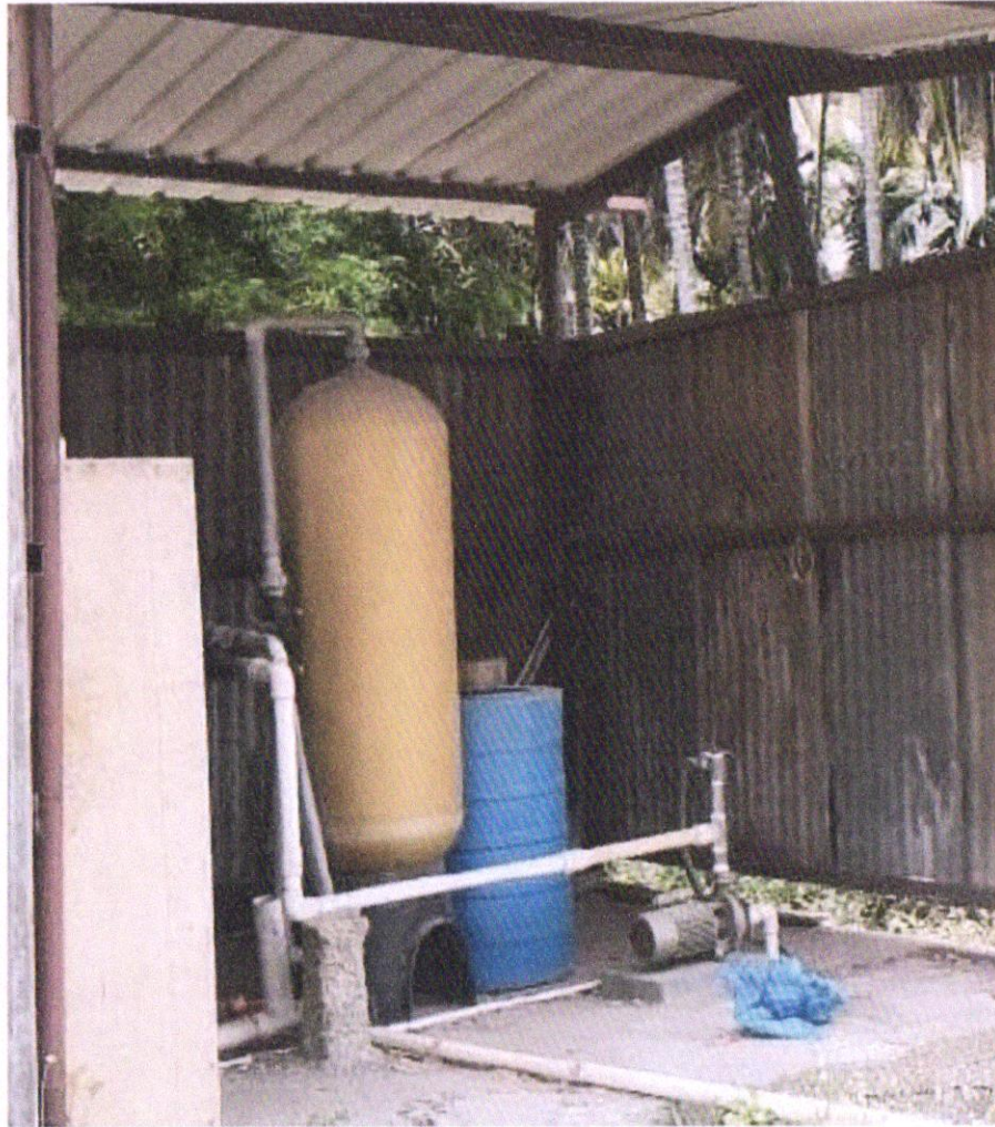
REVERSE OSMOSIS UNIT
